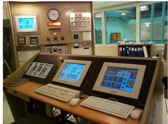
Fig. 2 View of reactor control room.
